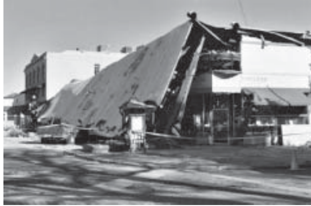
Paso Robles, CA January 25, 2004 — Structures and a vehicle damaged in downtown Paso Robles in the 6.5 San Simeon Earthquake. FEMA Photo/Dane Golden
